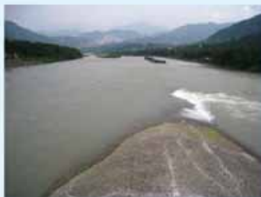
都江堰鱼嘴出现了裂缝 Cracks appear on the "Fish Mouth" of the Dujiang Irrigation System
